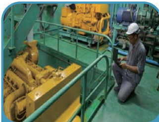
Engine Positioning Control Room
